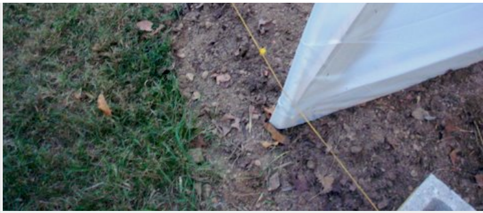
Once the end frames are in place pull a string to line up the stakes for the ribs.
