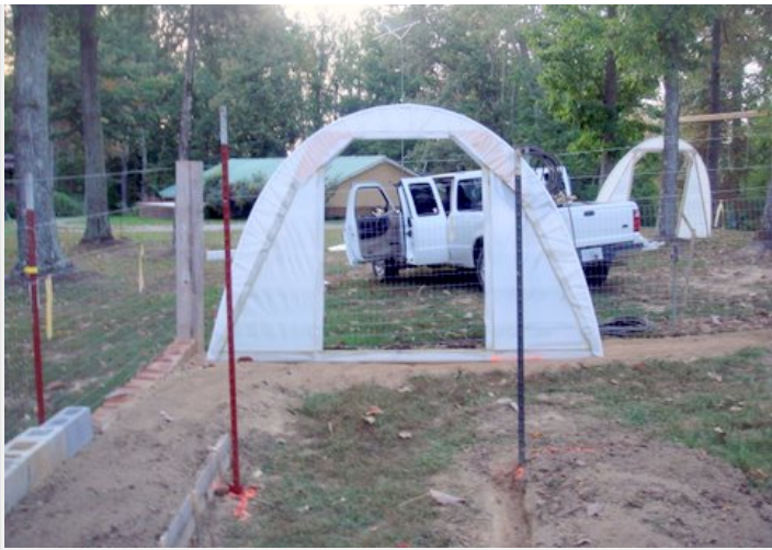
Mark out the locations of the door sides on the ground, and drive fence posts or long pieces of rebar at the sides of the door frame.
