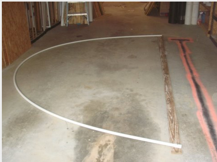
I temporarily attached a joint of pipe to a piece of 1x4 to establish the outline. You might be tempted to make your greenhouse wider and lower at this point to get more floor space out of it - but be careful. If you have snow in your area it will slide off of a high peak a lot better than it will if your greenhouse has more of a flattened shape - and the same goes for heavy rains. If your greenhouse is too flattened it will cave in the first time it snows or rains really hard!
